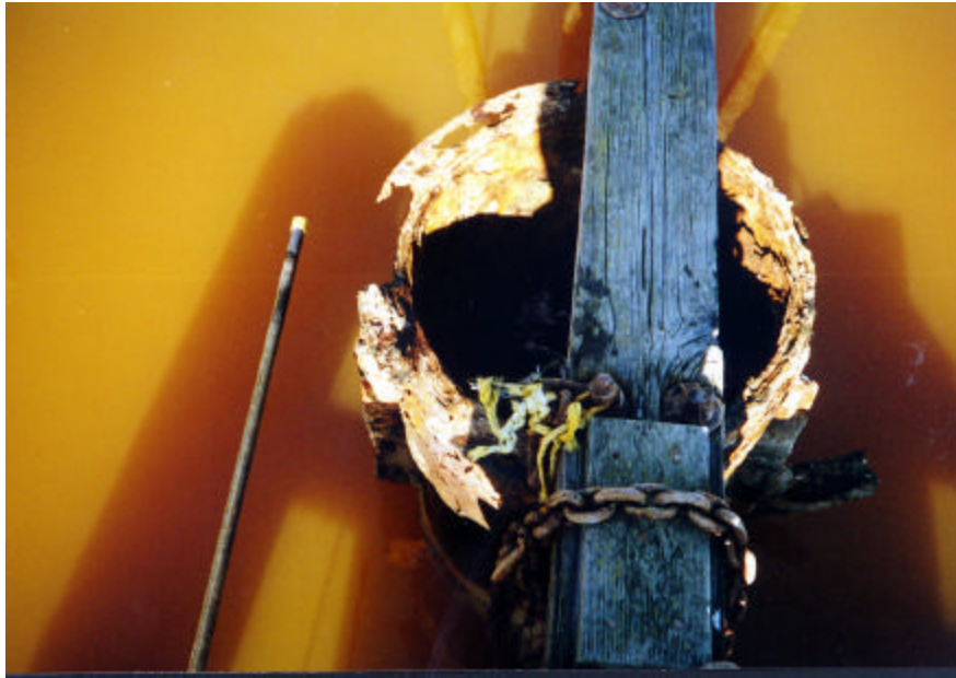
The acoustic velocity recorder was fixed into the invert of the siphon using an access shaft for each of the siphons measured
